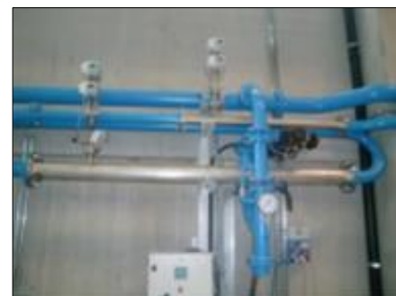
2 measuring tubes (stainless steel) DN 80 and DN 150 with two PoetterSensors® and two DP- Transducers for each pipe
